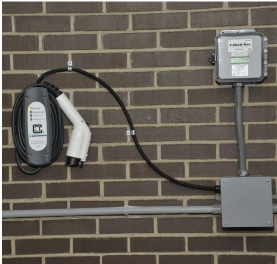
Wall-mounted Level 1 EVSE used for workplace charging (New York Power Authority Photo)
