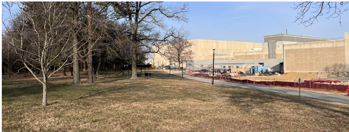
Museum Support Center Pod 6 Construction underway at the Suitland Collections Center will reduce risks to collections stored at museums in the 100-year flood plain.
